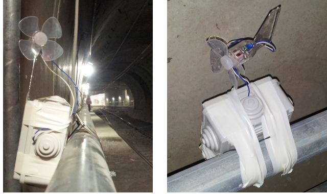
Figure 3.5: Snapshot of nodes deployed in a tunnel of the Metro B1 line in Rome.
